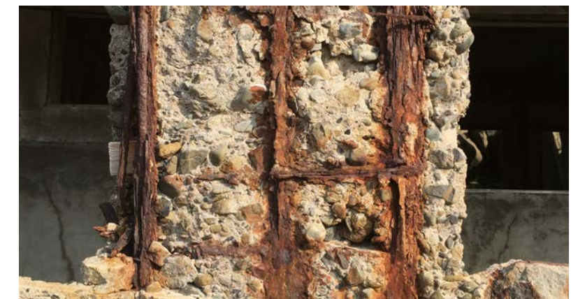
Rust formed on steel bars embedded in concrete. Corroded steel bars expand, causing the surrounding concrete to crack.
